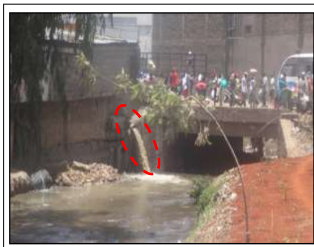
Plate 5.5: Direct Discharge of Raw Sewerage into the River
