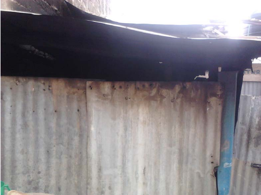
Poorly ventilated kitchen
