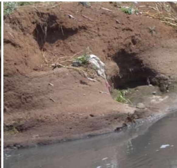
Plate 4.2 f: Undercutting of inner bank/pop out failure results to cavities
