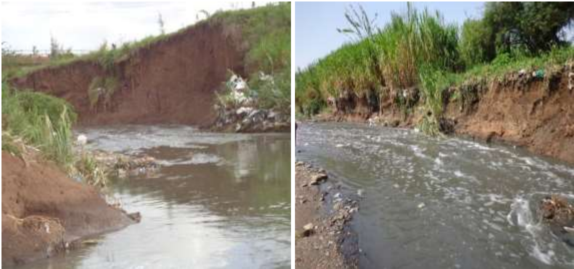
Plate 4.2 c: Land slide of high river cliffs Plate 4.2 d: Collapsing of banks
