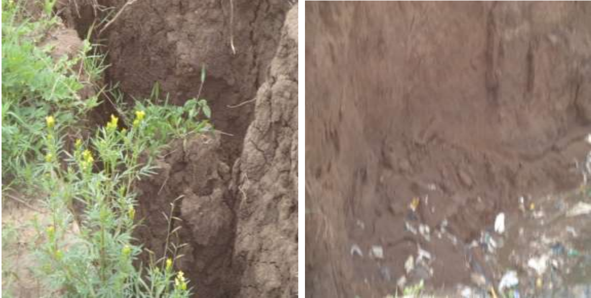
Plate 4.2 g: unstable outer bank showing cracks Plate 4.2 h: collapsed outer bank
