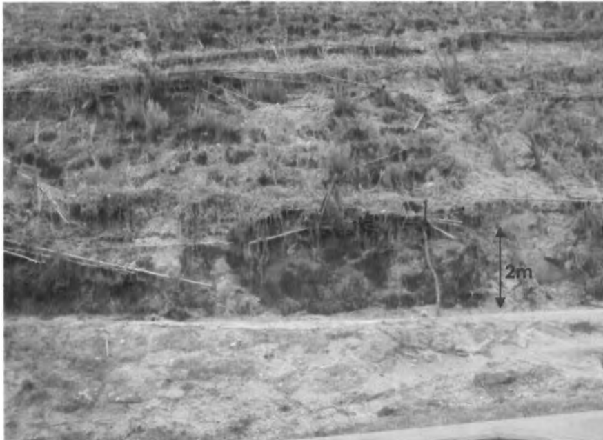
Fig. 3.2: Photograph of the research site showing an eroded terrain with effects of shallow landslides in which the sliding surface is located within the soil mantle or weathered bedrock (typically to a depth from few decimetres to 1 metre)
