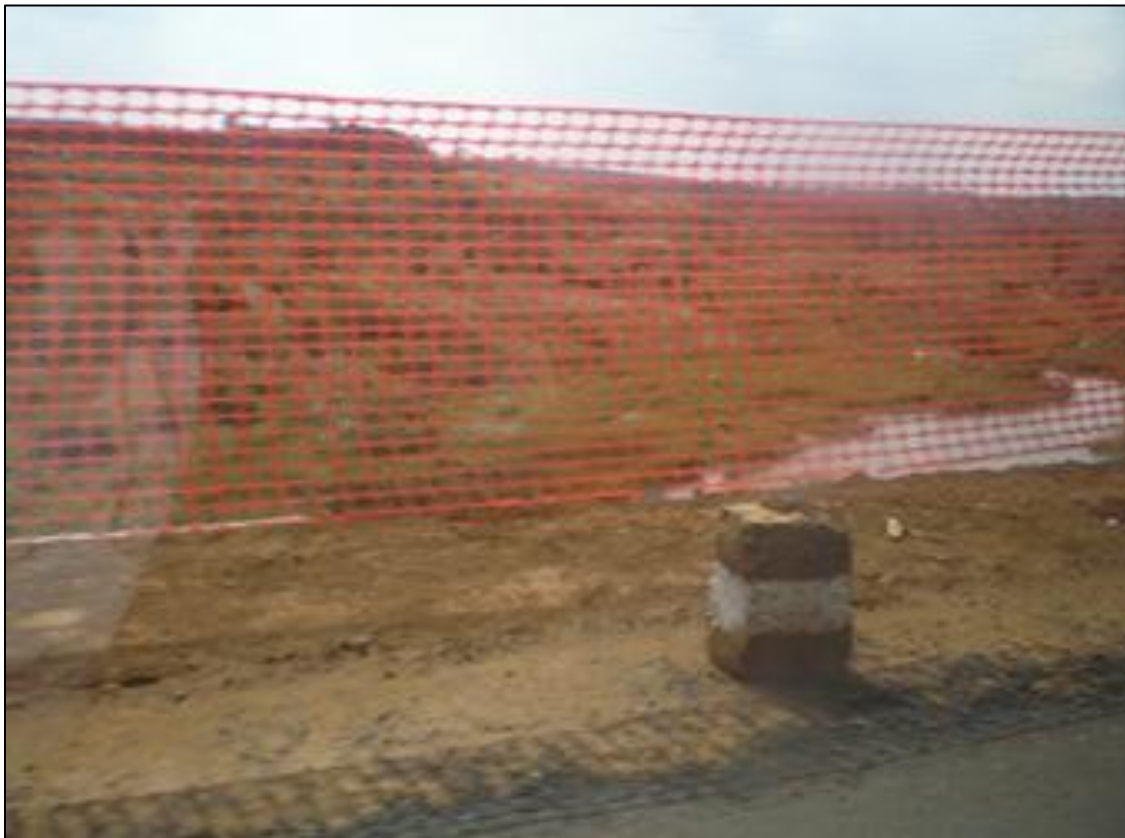
Plate 6: A Blocked river channel on Lot 3 of Ruiru River with potential impact of affecting aquatic life forms
