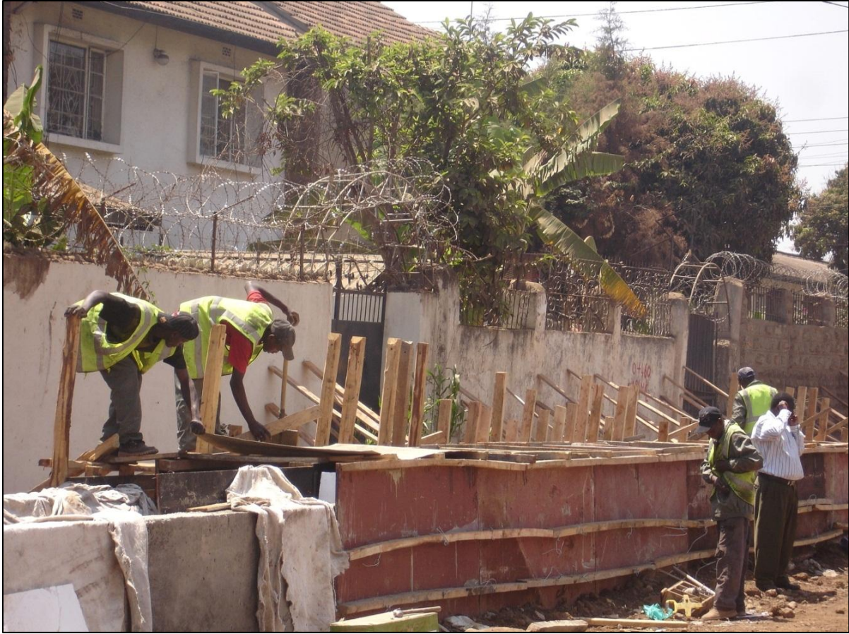
Plate 20: Note: the construction of one of the open drainage systems at Pangani area (Lot 1)
