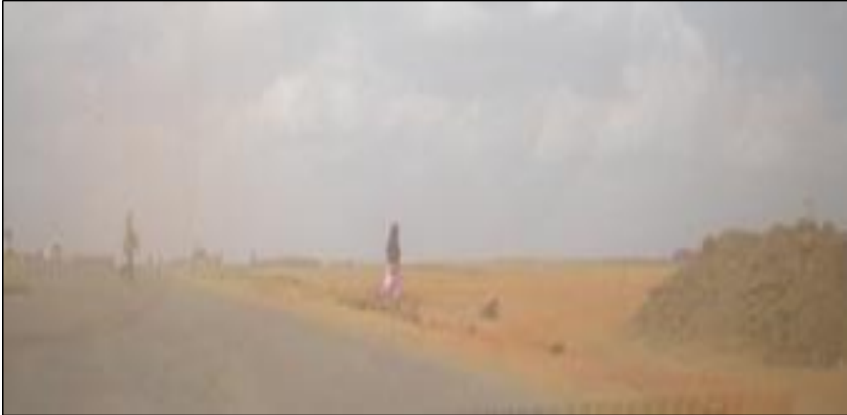
Plate 14: Clouds of dust emissions from road construction works with potential impact on human health on Lot 3 at Kenyatta University
