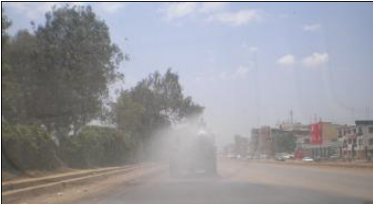
Plate 17: Road construction workers spraying water on the road to keep down dust on Lot 2 (Kasarani area)
