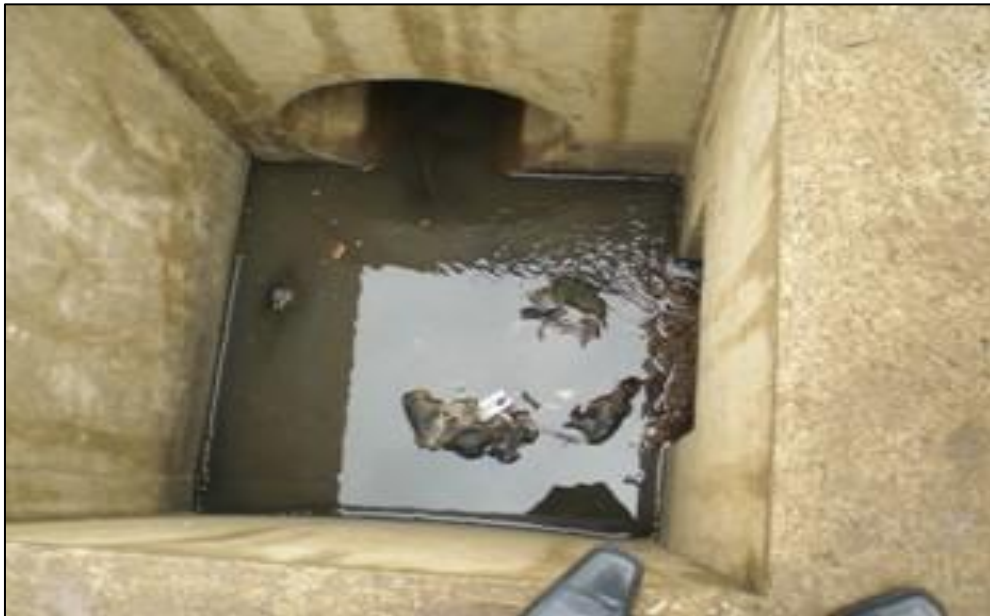
Plate 5: Uncovered culvert along the University Way posing risks to the pedestrians
