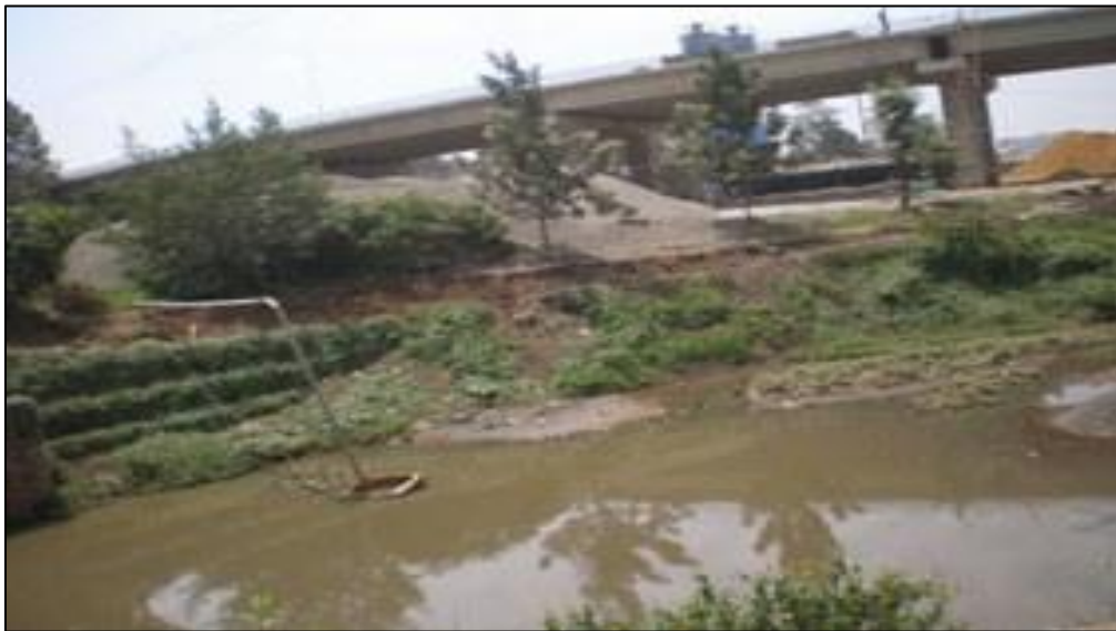
Plate 4: Severly degraded Nairobi River channel at globe Cinema round about
