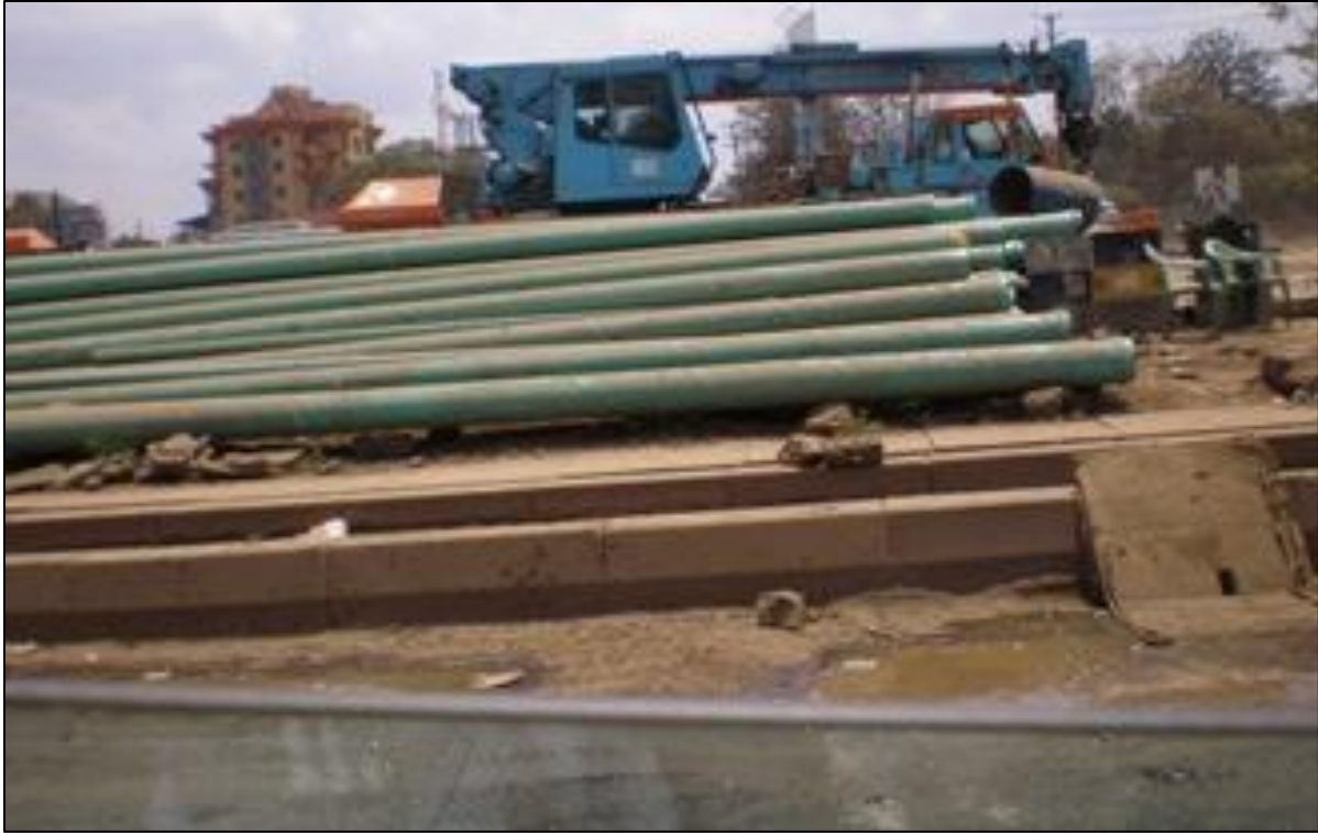
Plate 18: Construction materials stored on the road side posing risks of theft and accidents
