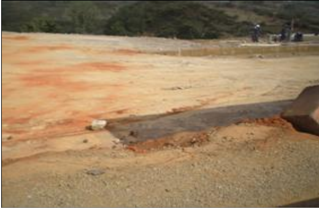
Plate 5: A Section of the road on Lot 3 which will directly impact the riparian vegetation health
