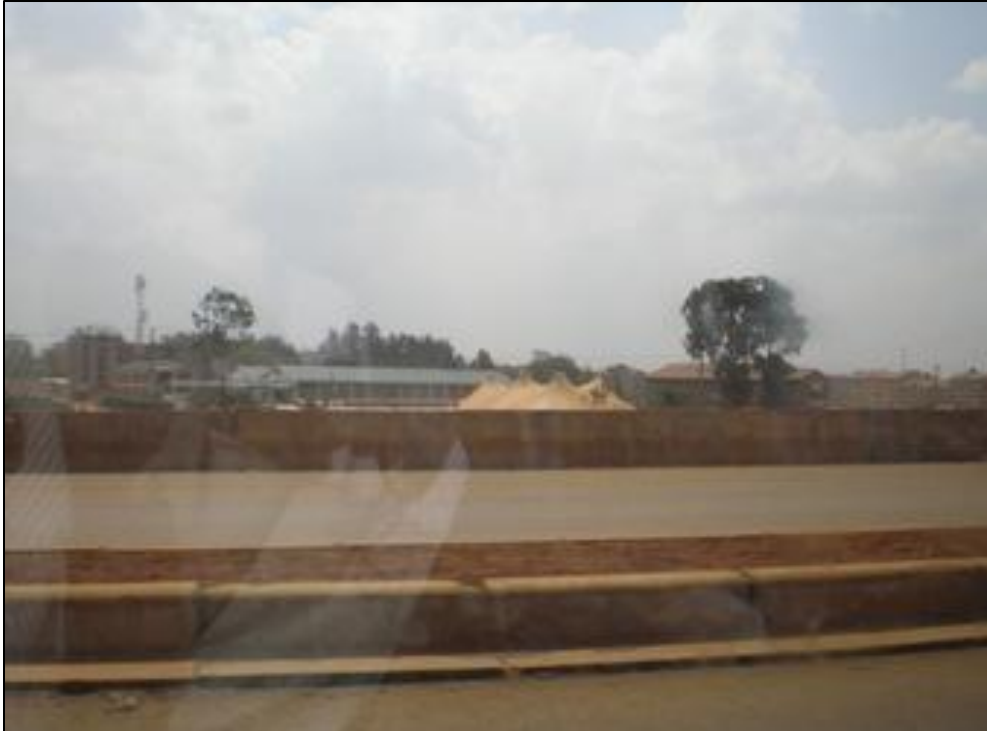
Plate 16: Dust emissions from the road construction settling on the neighbouring buildings with potential negative impact on air quality
