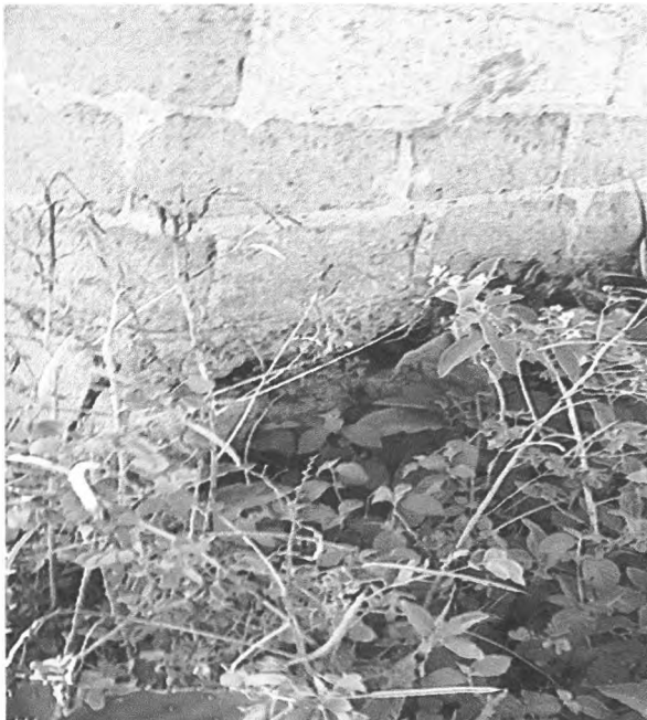
Photo 4.5: Pit latrine wall beginning to crack near the ground in Wandiege
