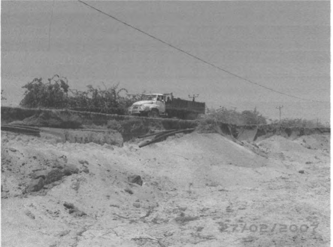
Plate 12: Destruction of roads, water pipes, telephone and electricity lines
