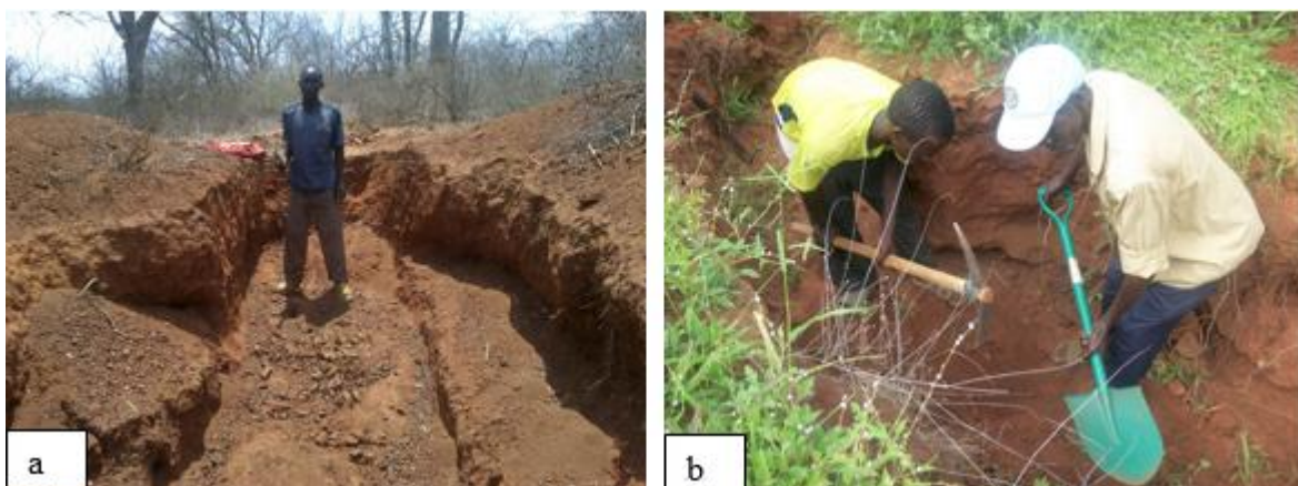
Figure 3.8. Pitting and trenching to collect samples in Mutuluni (a) and Katokolo (b) areas, east of Ikutha town.
