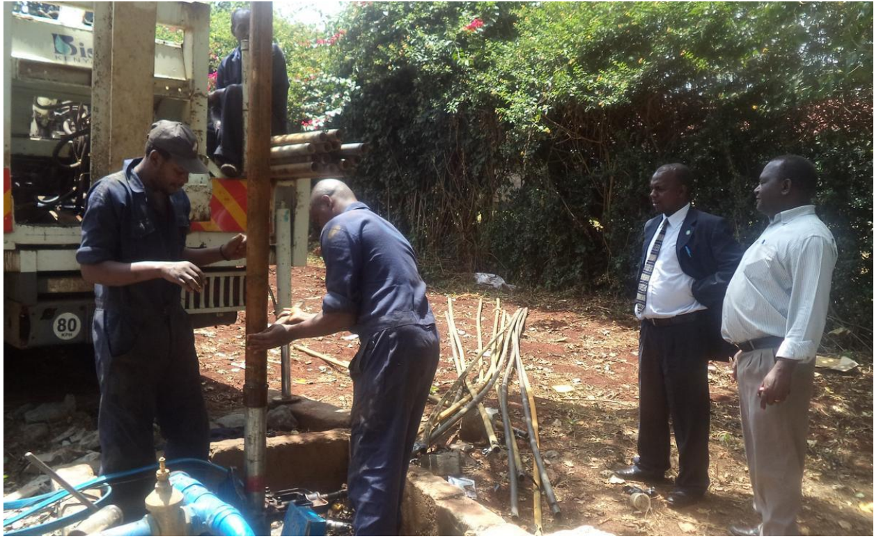
School of Business inspects the borehole water system at lower Kabete campus.
