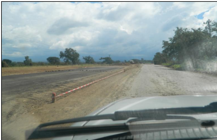
Plate 14: The road to the Mt. Kenya National Park gate from Narumoru Town currently under being tarmacked
