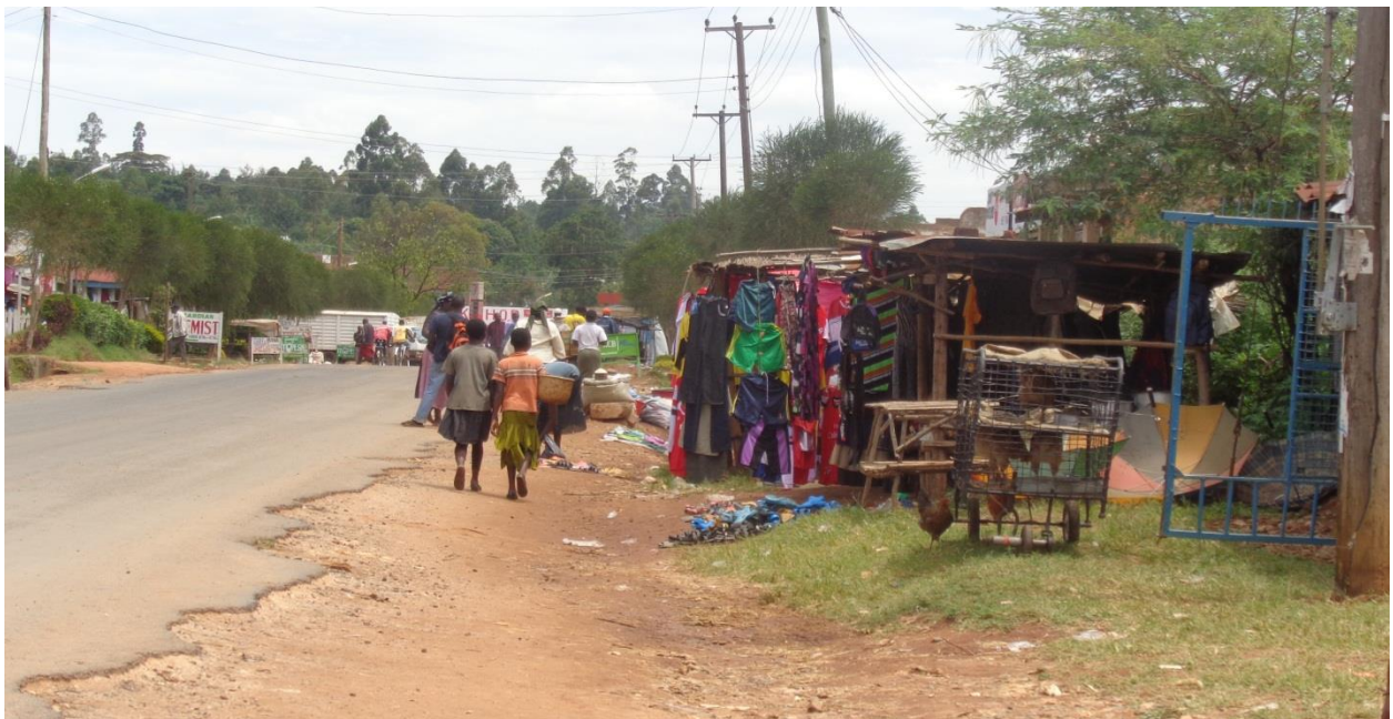
Plate 4.11: Tarmac Surface Peeling Off
