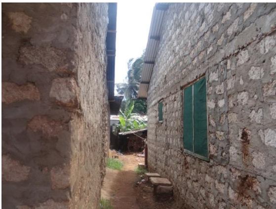
Poor building standards
