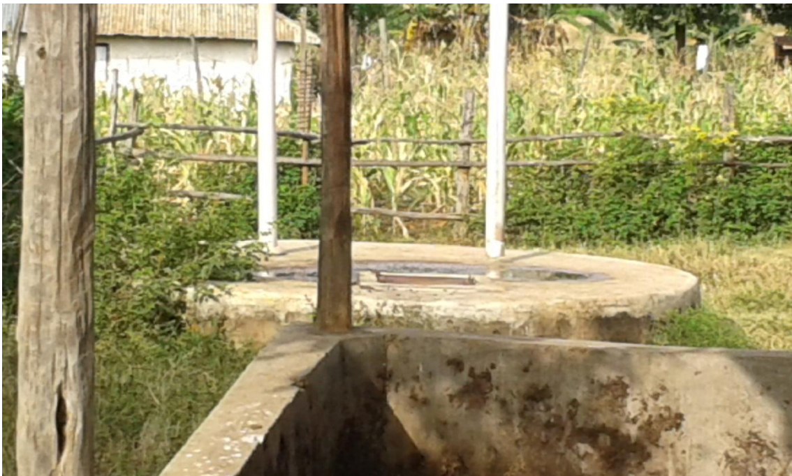
Condemnation pit in Sagana slaughterhouse
