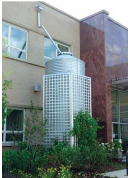
Figure 9: Rainwater storage tanks to store rainwater for reuse (Source: Chicago's Water Agenda, 2003)
