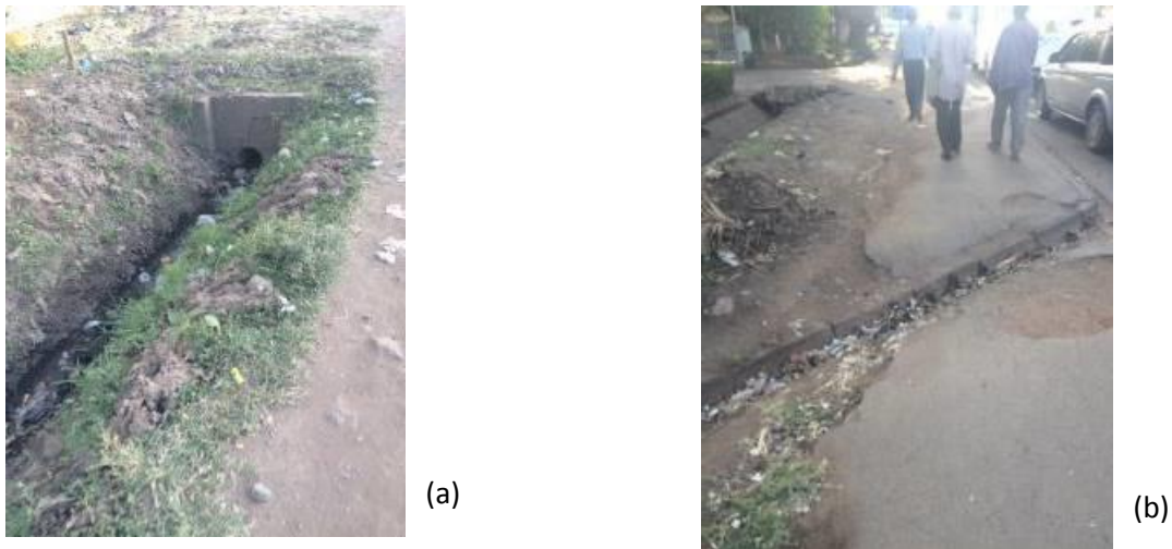
Figure 27: Pinch point (a) and Drain channel in poor condition (b)
