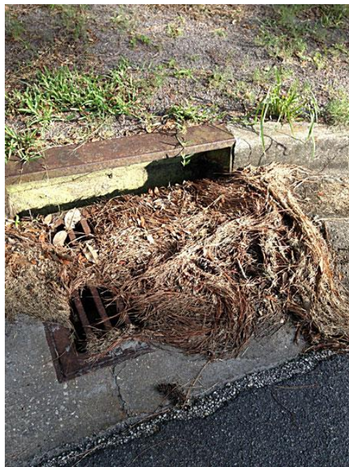
Figure 6: Debris blocking a storm water inlet drain (Source: Author)
