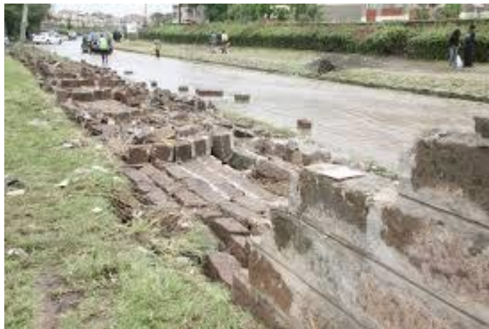
Figure 3: Damaged boundary wall as a result of floods in Midlands Estate, South C. (Source: Daily Nation, 18 th October 2014)
