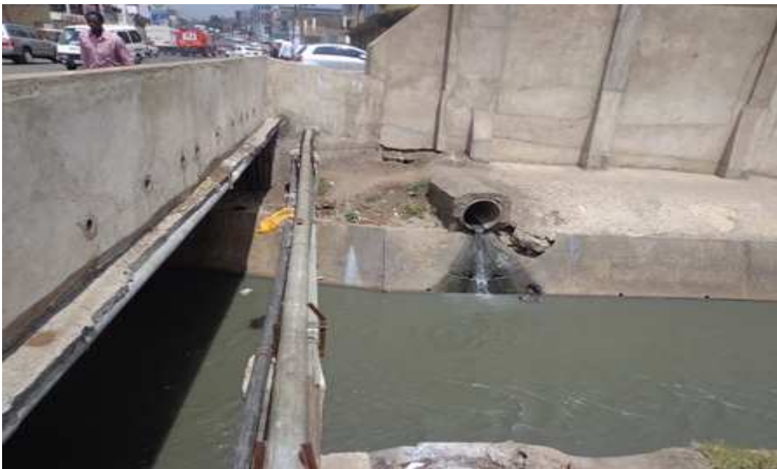
Plate 10: Ngong River across the Mater Hospital Bridge. Notice the direct sewer discharge from some section of industrial area.
