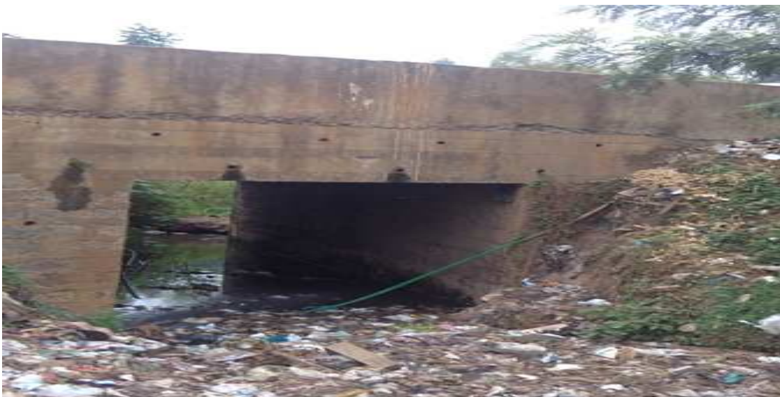
Plate 4: Jamhuri Dam outlet just after Kibera Bridge. Here, clear water just before the Bridge is contaminated with solid wastes dumped by Kibera residents and a stream of sewerage from the slums at the bridge.
