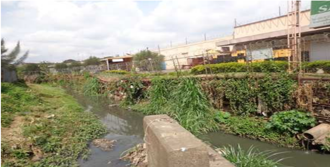
Plate 9: Ngong River crossing Nairobi West. Notice the direct sewer discharge at the Nairobi West mall.
