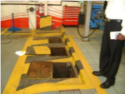
Plate 3: Oil/water separator at Toyota Kenya Workshop
