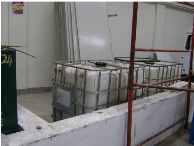
Plate 7: Accidental spillage containment structure at RMA Motors (K) Ltd
