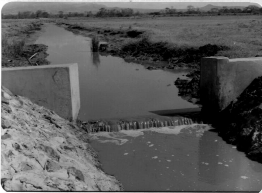
Fig.4.4: Old Kimorigo drain at head of scheme. In the photo is a measuring weir under construction. (Photo taken end of March before floods).
