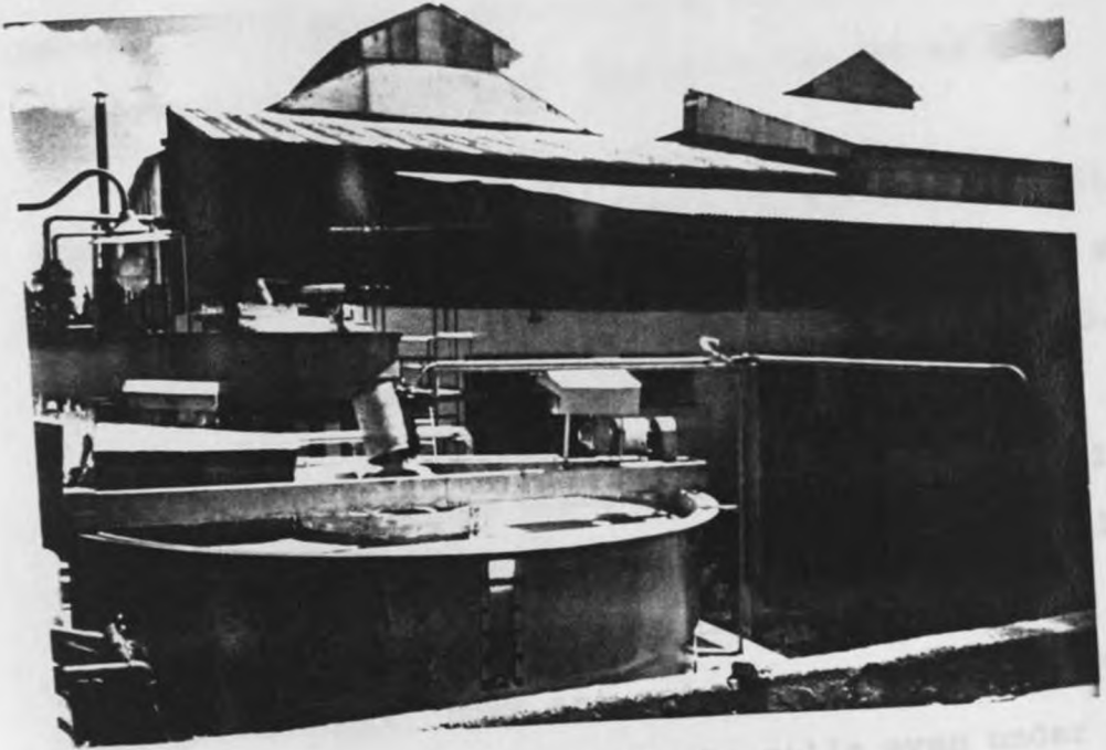
PLATE 4.1 PM1 and PM2 Clarifiers (Krofta Treatment Plant)
