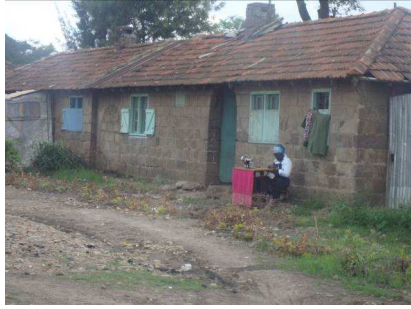
Plate 49. Poor state of buildings
