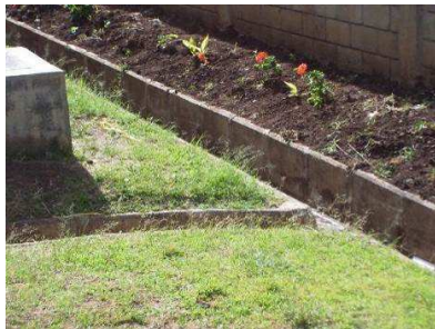
Plate 19: On surface stormwater drainage
