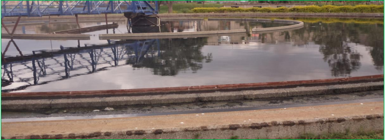
Figure 2.7: Kariobangi Treatment Works Clarifier
