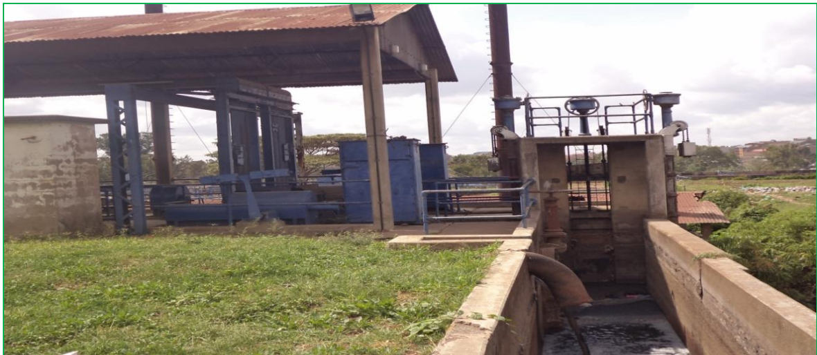
Figure 2.6: The Kariobangi Treatment Works Inlet
