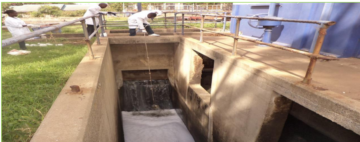
Figure 2.10: The Kariobangi Treatment Works outlet
