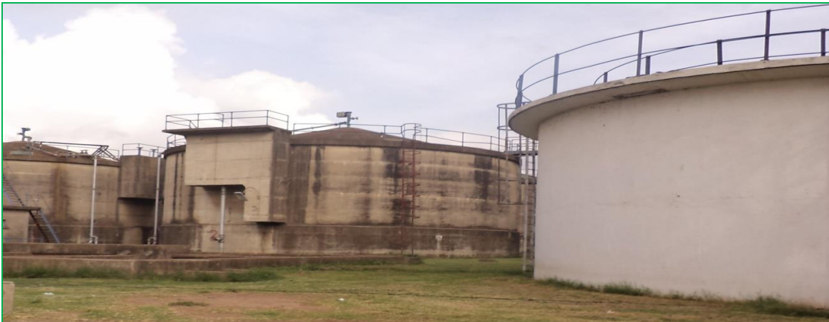
Figure 2.8: Sludge Digestion Tanks at Kariobangi Treatment Works
