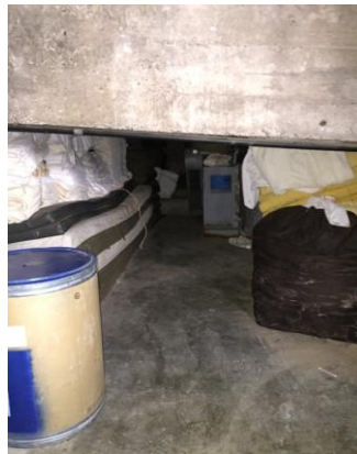
Plate 20: Low Ceiling in Plant Room
