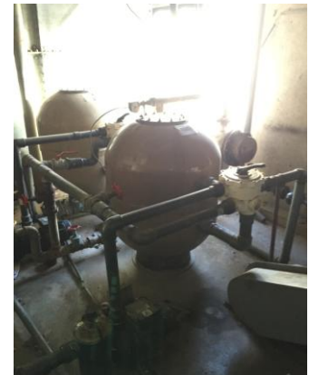
Plate 21: Swimming Pool Pump Room
