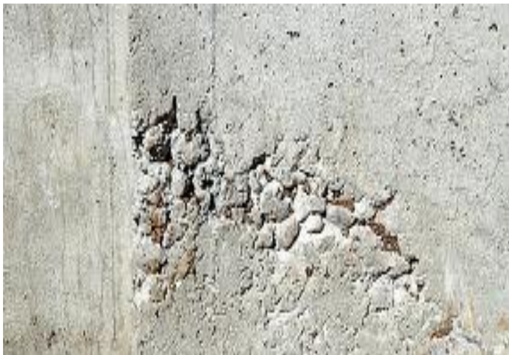
Plate 2.3: Honeycombing on a concrete surface
