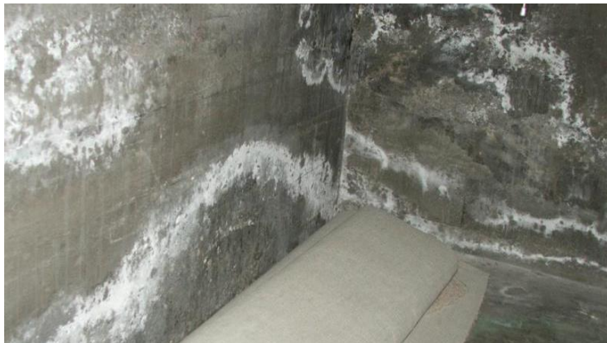
Plate 2.7: Efflorescence on concrete surface
