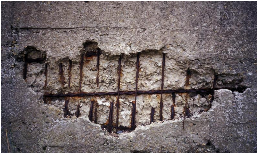
Plate 2.9: Corrosion of reinforcements
