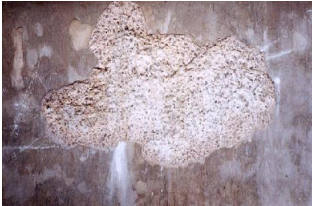
Plate 2.2: A Spalled Concrete Surface
