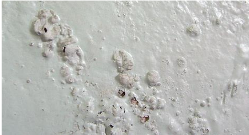
Plate 2.8: Blistering on concrete surface
