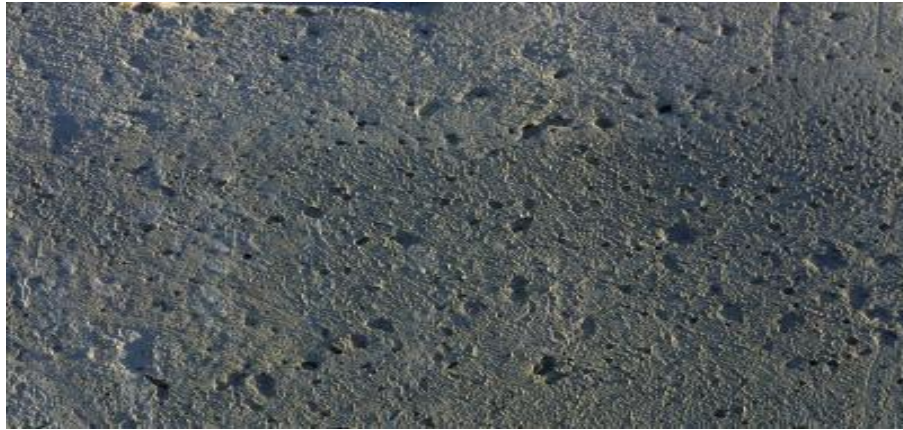
Plate 2.6: Concrete surface which has been damaged by rain
