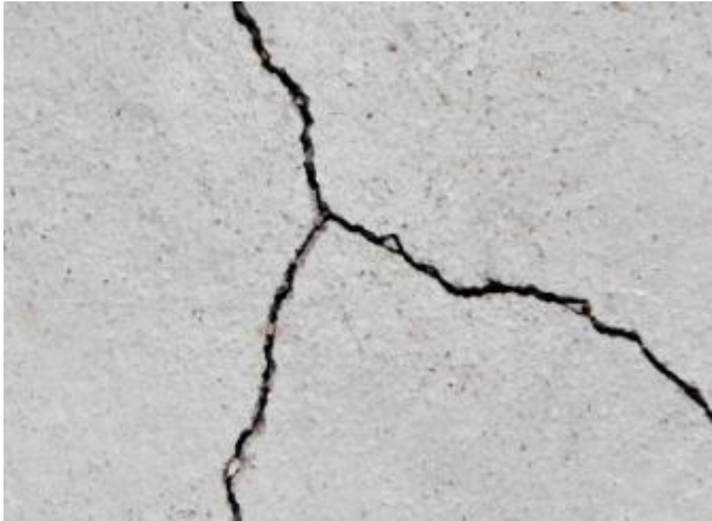
Plate 2.1: A cracked concrete surface
