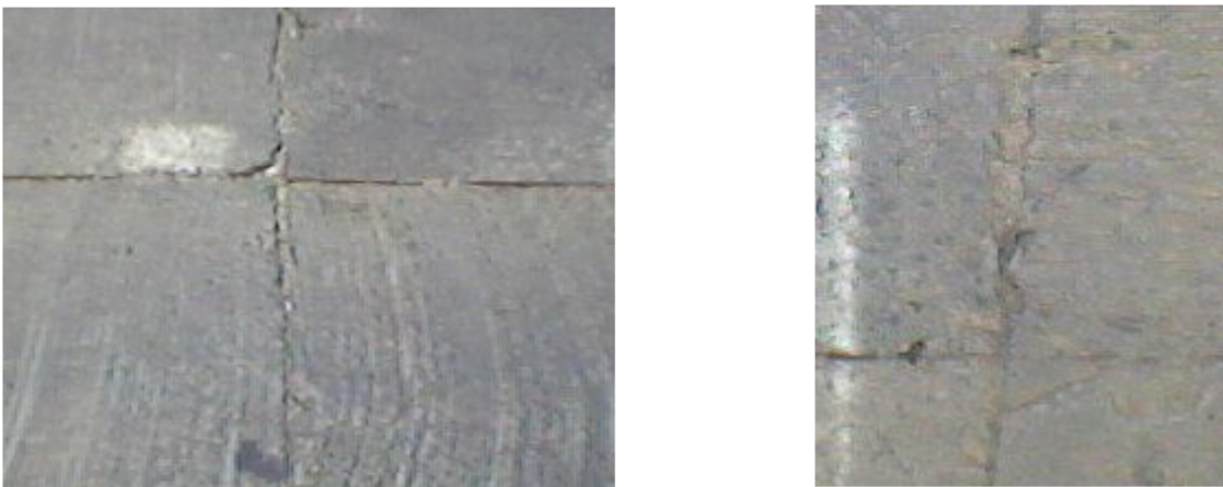
Fig 4.1: Joint spalling at chainage 2450m
