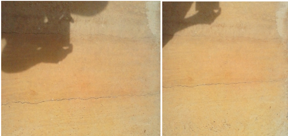
Fig 4.11: Major transverse cracks across the beam
