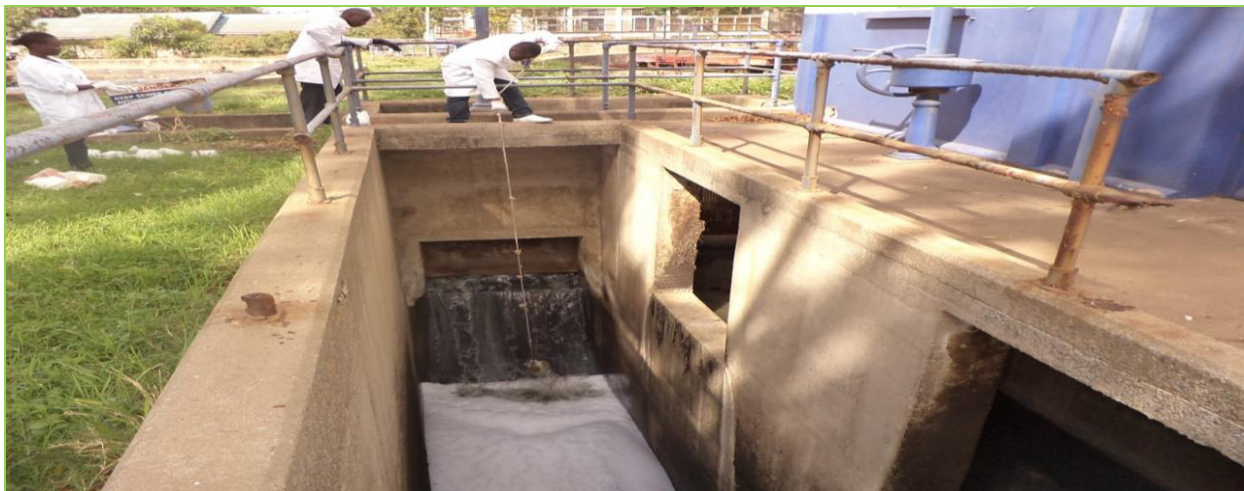
Figure 2.10: The Kariobangi Treatment Works outlet
