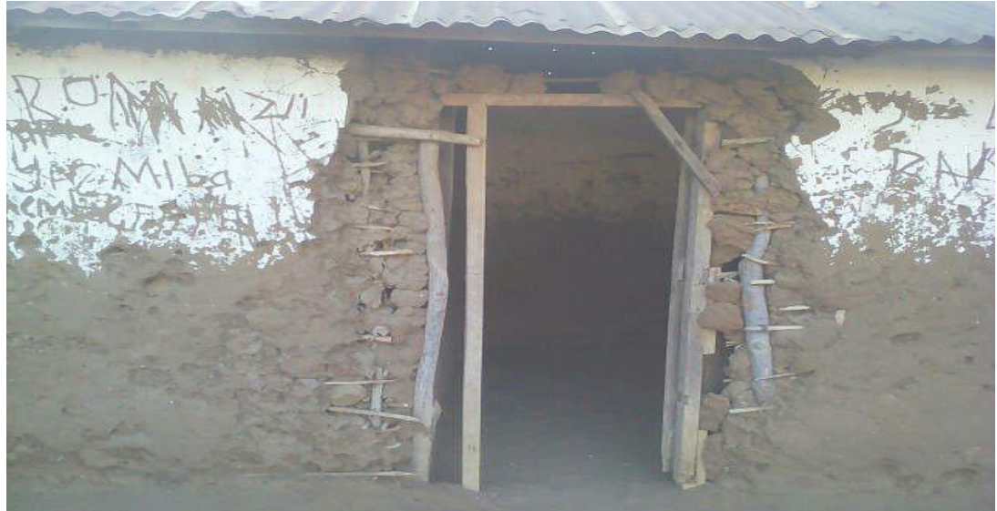
A semi-permanent building of Madrassatul – Tawakal of Makere village in Galole constituency
