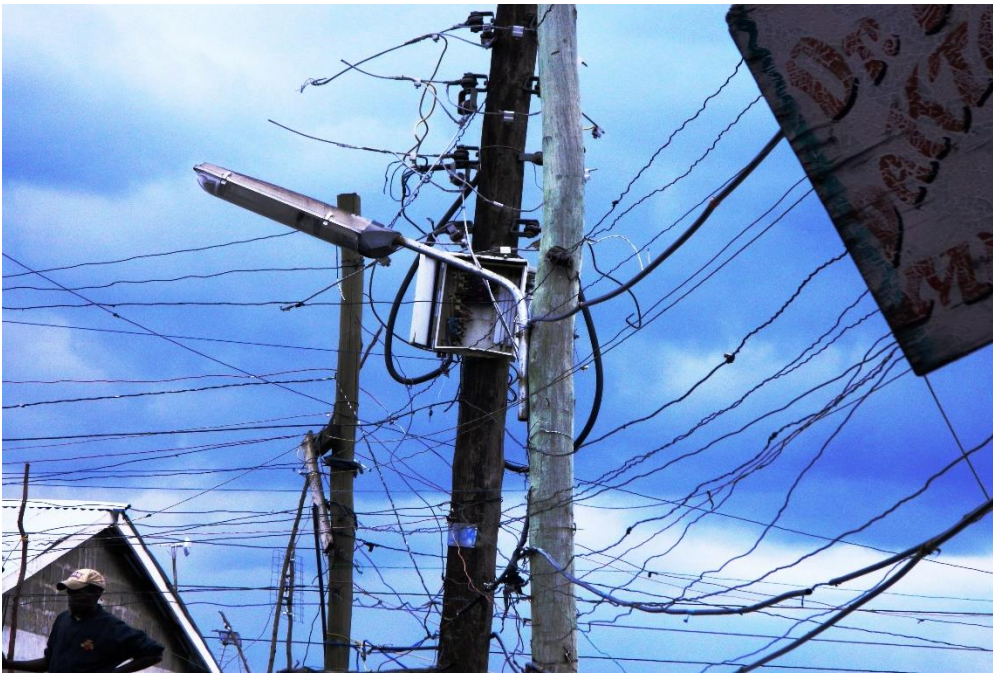
Photograph 3: Illegal Electric Connections in Mukuru
