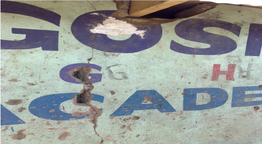
3 Classroom wall: exhibiting cracks on wall and gaping holes posing a hazard to the students.
