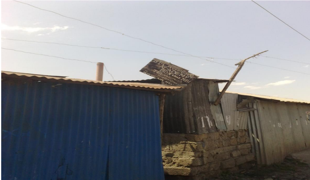
5 School entrance: exhibits precariously hanging electric cables at the entrance of the school
