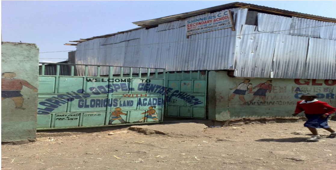
1 Photo of a school entrance: exhibiting precariously hanging iron sheets used as class wall and loose electric cables next to them.
