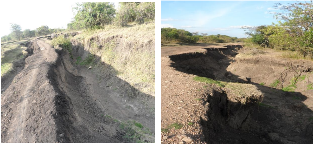
Plate 4.4: Dilapidated roads within the conservancy
