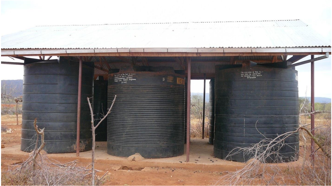
Water tanks protected four years after the emergency
