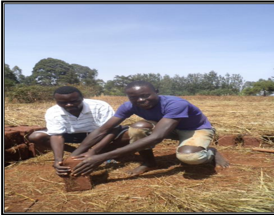
Plate 5 is a photograph captured in Kakamega North in 2012 displaying the investigator arranging raw bricks at a working site.
