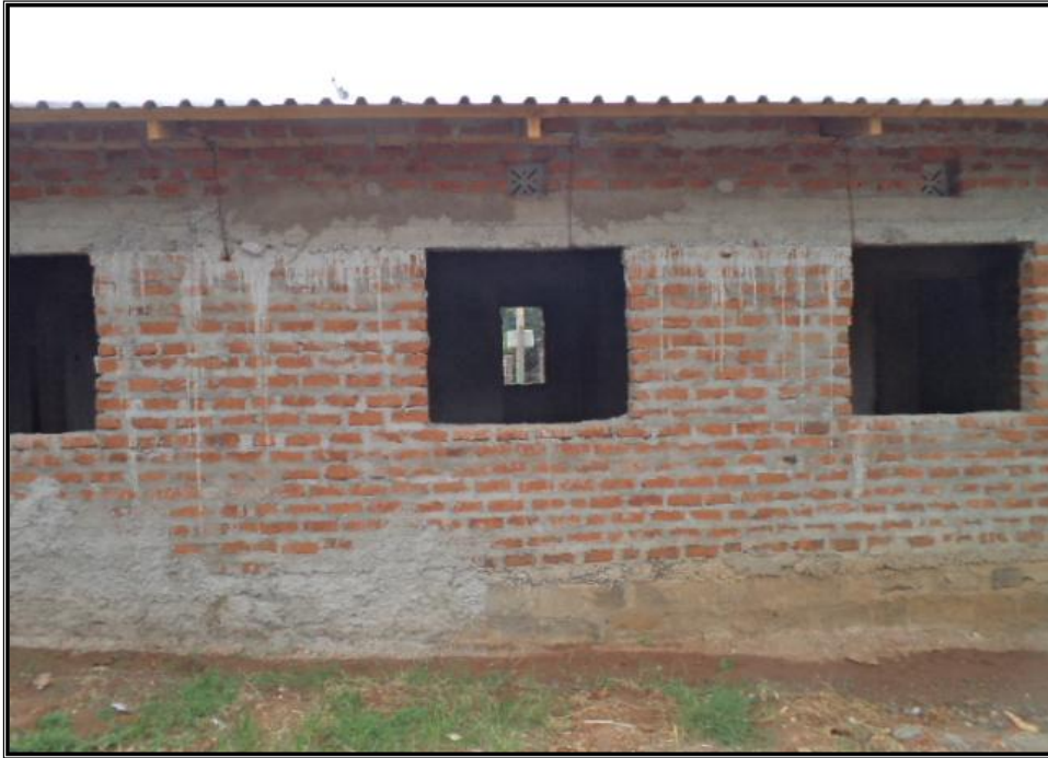
Plate 6 is a photograph captured in Lugari in 2012 (by the investigator) displaying a brick-walled house under construction.
