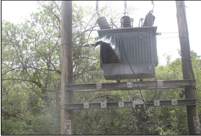
Plate 5.5: Exploded transformer that has not been repaired for over one month
