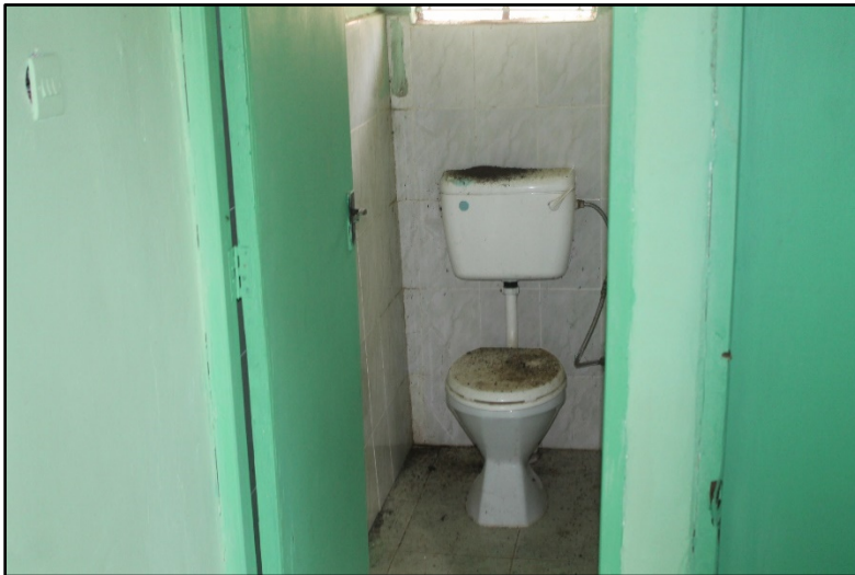
Plate 5.2: Abandoned toilet facility
