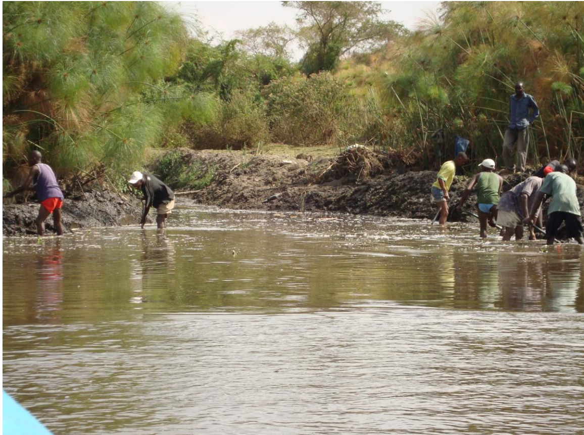
Plate 2-2: Canal dredging and repair works in the southern zone of Lake Naivasha (Researcher 2009)
