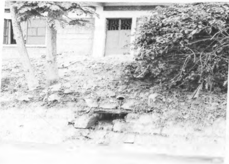
Plate 4.23: Structure Built on top of a Sewer in Dandora Area 2 (Note the raw sewer discharge into the open drain along Apudo Road)
