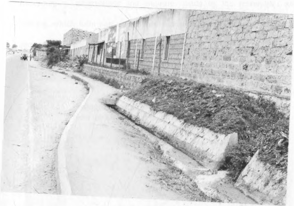
Plate 4.14 Illegal Constructions on a Road Reserve (Southern Access Road)
