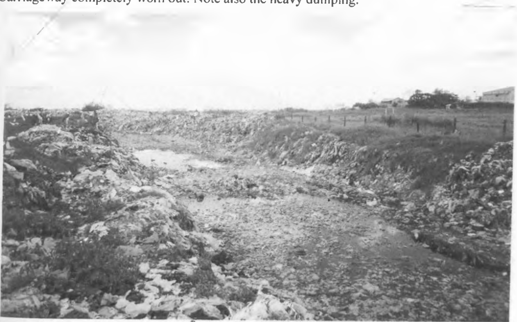
Plate 4.11: Remains of Northern Spine Road in Area 6 Carriageway completely worn out: Note also the heavy dumping.
