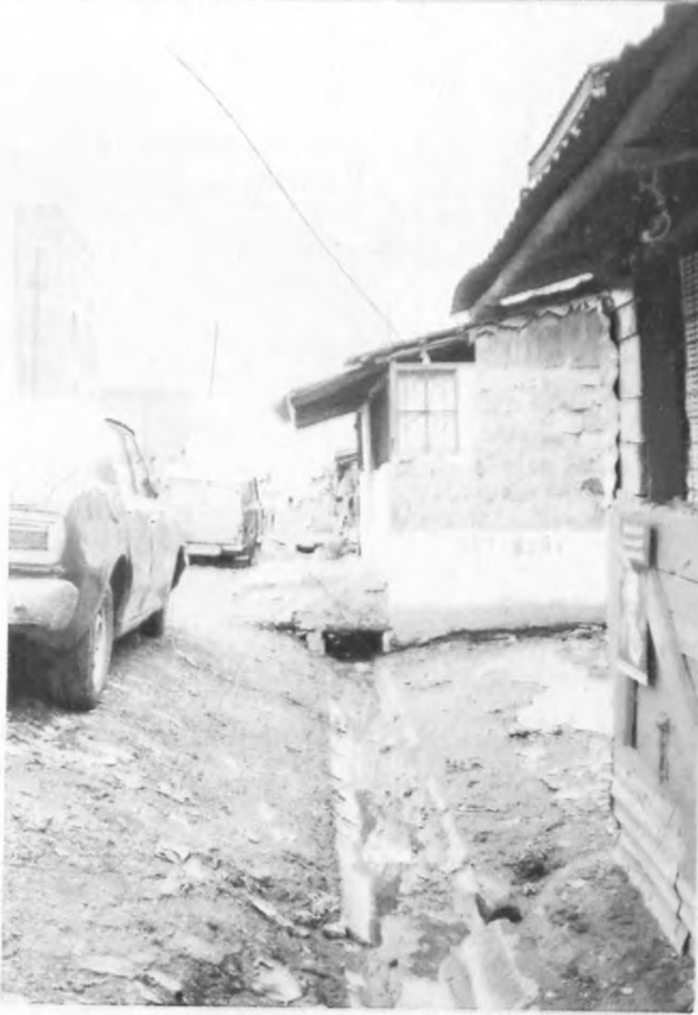
Plate 4.19: Obstruction of Storm Water Drain by a Kiosk (Note also the silting)
