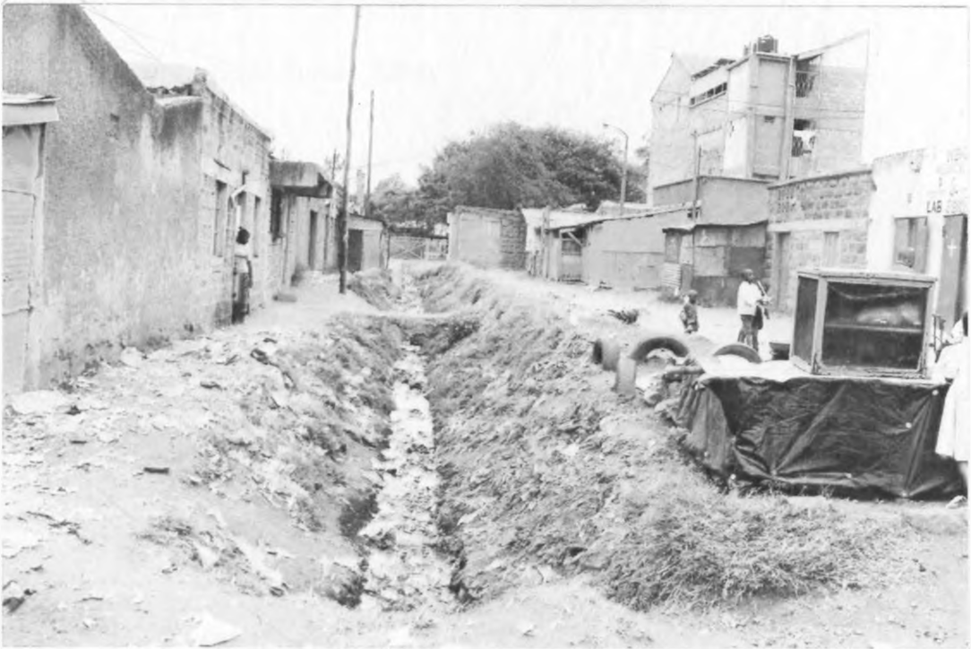
Plate 4.18 Storm Water Drain Covered by Vegetation in Dandora Phase I
