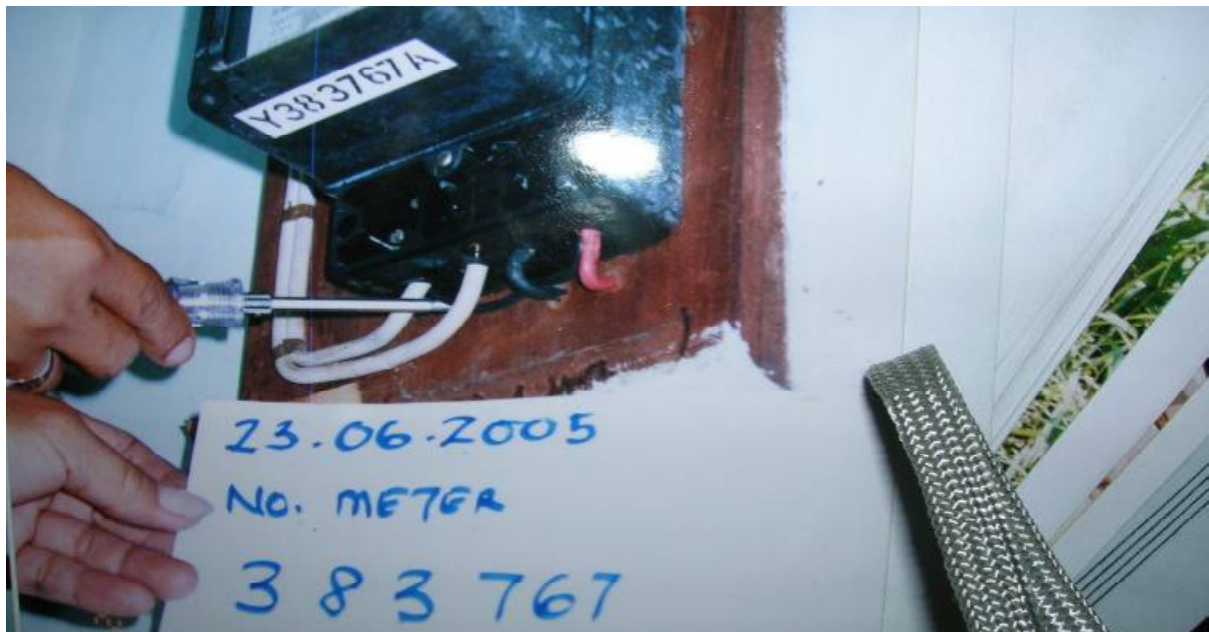
Figure 2.7: A photograph showing a tampered energy meter.
