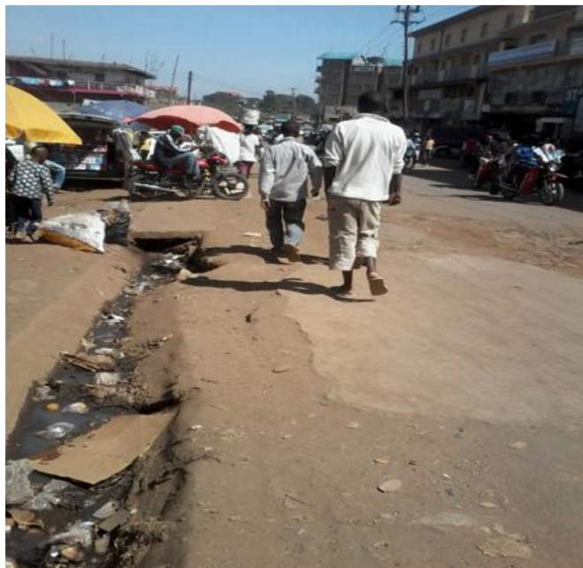
Plate 5. 9: Blocked Storm Drains
