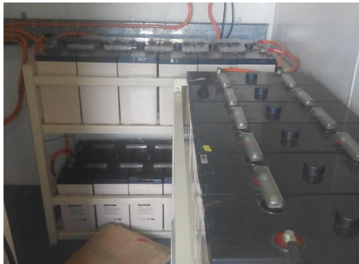
Figure 4: Battery Unit (Storage Power) 24 batteries as configured in the site
