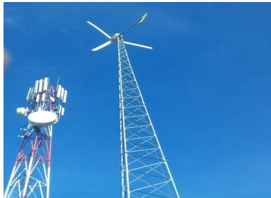
Figure 2: Wind Turbine and Communication Mast
