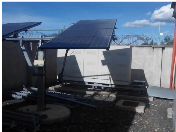
Figure 1: Solar Panel mounted on the ground
