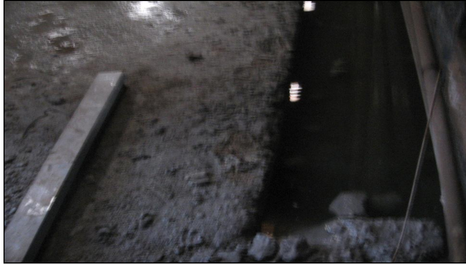
Figure 3.1: Sludge deposit next in the vicinity of the wastewater treatment plant
