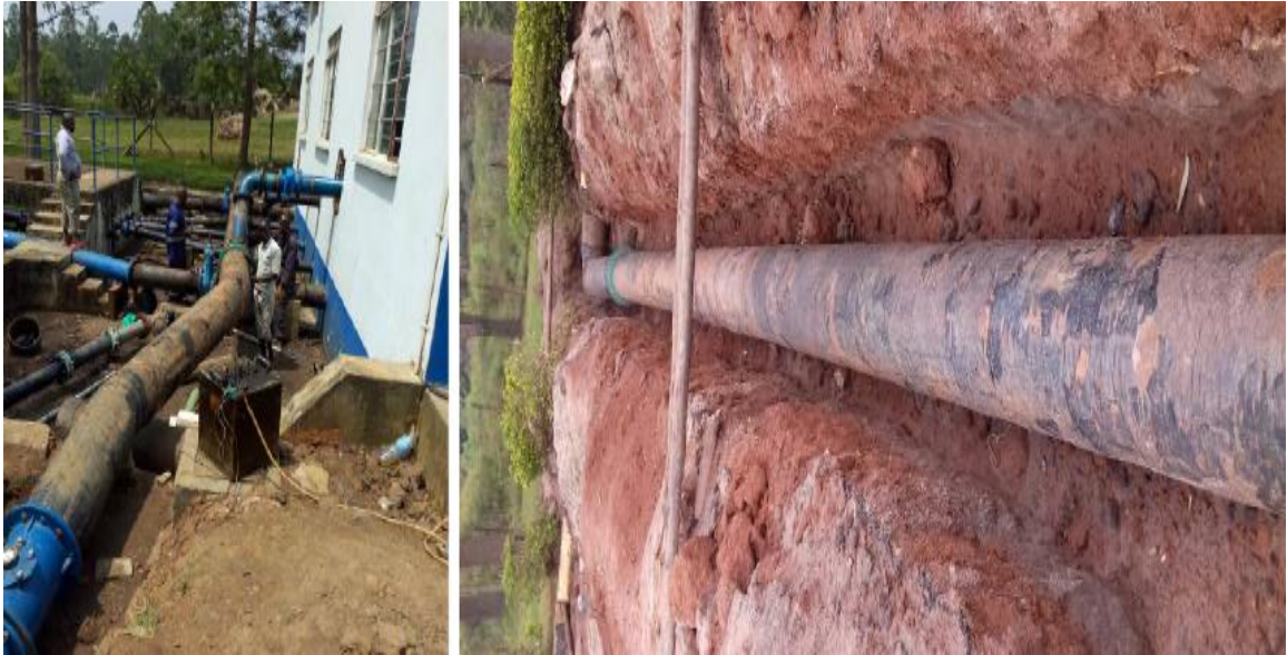
Plate 4.3: Showing NWSC Old Network Being Repaired at Ruharo Water Treatment Plant in Mbarara Municipality
