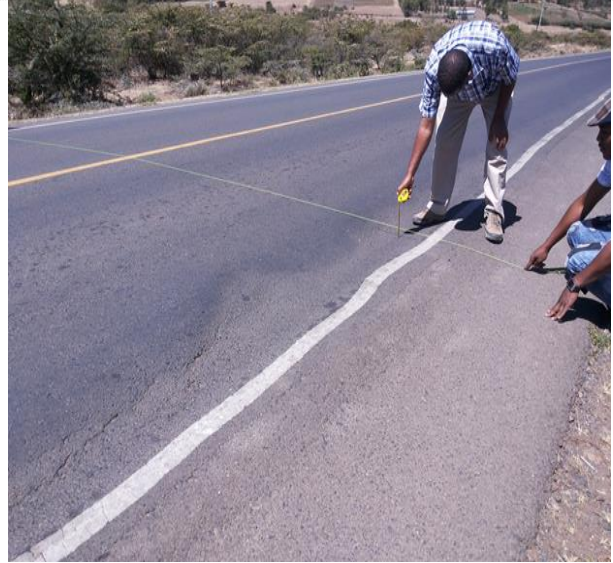
b- Rutting on LHS at chainage 50+000
