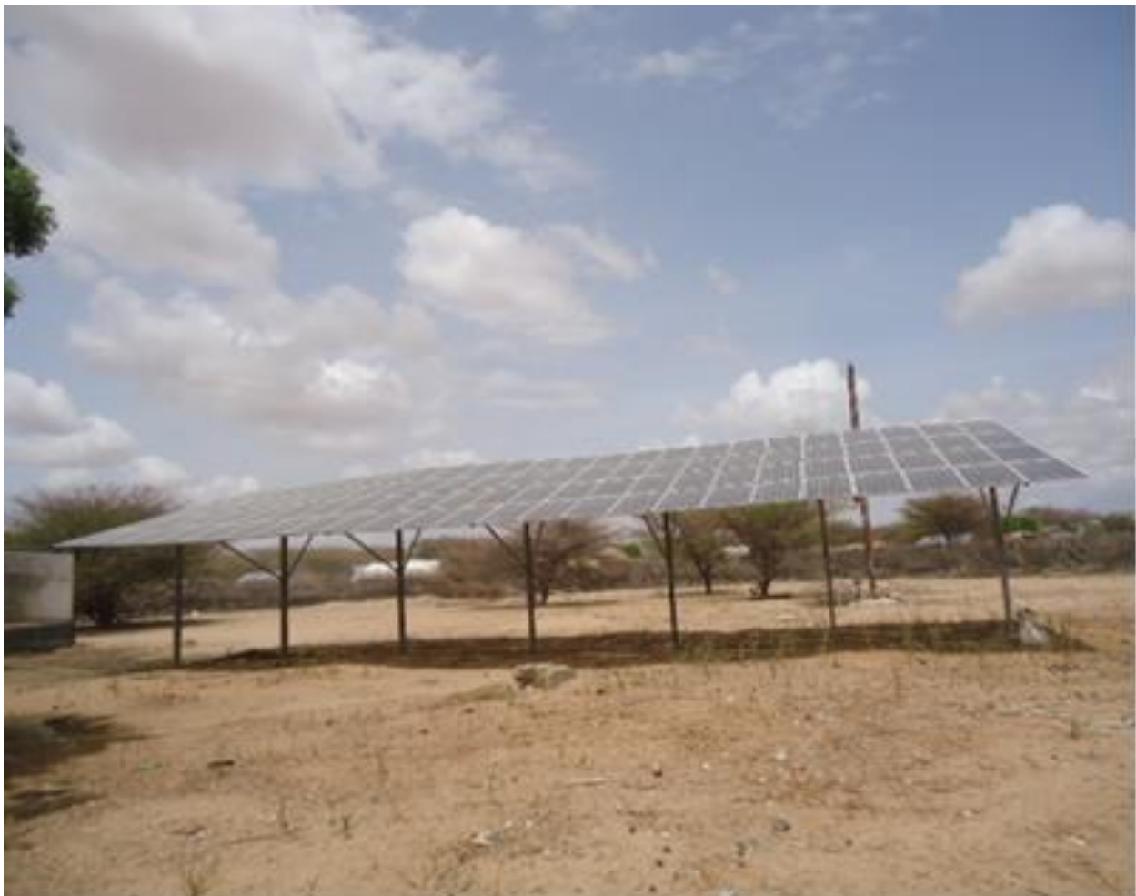
Figure 3.2: Solar water pumping system installed at Abakore
