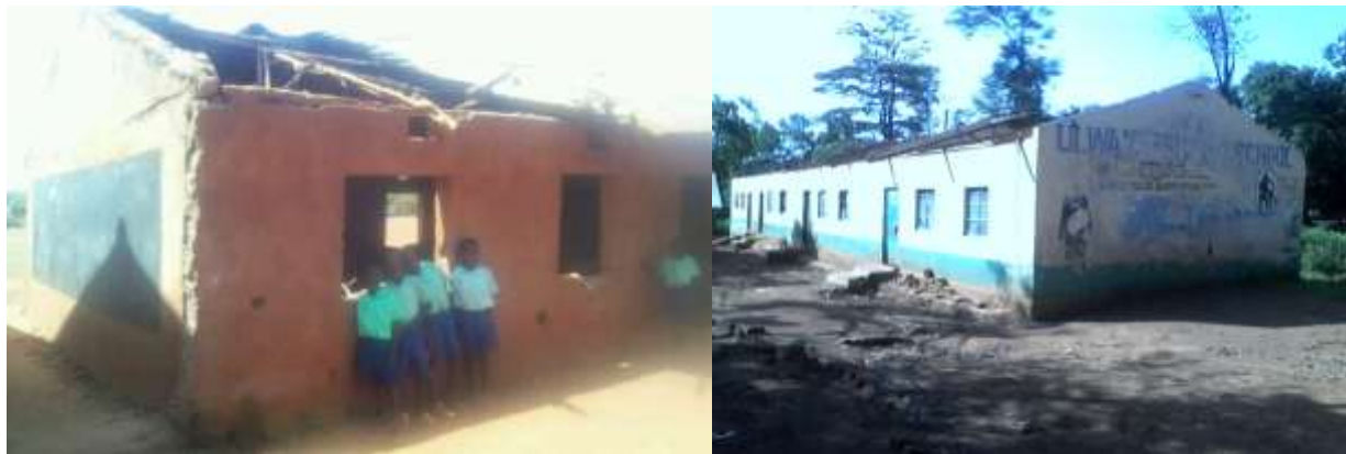
(a) Classroom roof of Sikalame primary school (Ugunja) (b) Ulwani Primary school (Ugunja) destroyed by windstorm ( source, author, 7/12/2017, 3.34 p.m.)
