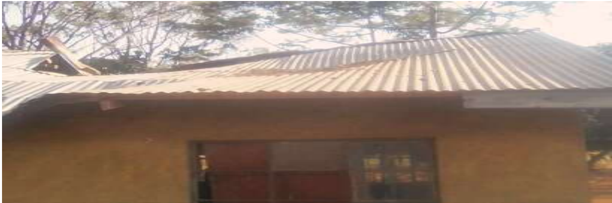
Figure 4.31: (c) Classroom roof of Umer Primary school (Ugenya) destroyed by windstorm (Source, author, 2/6/2017, 4.00 p.m.)
