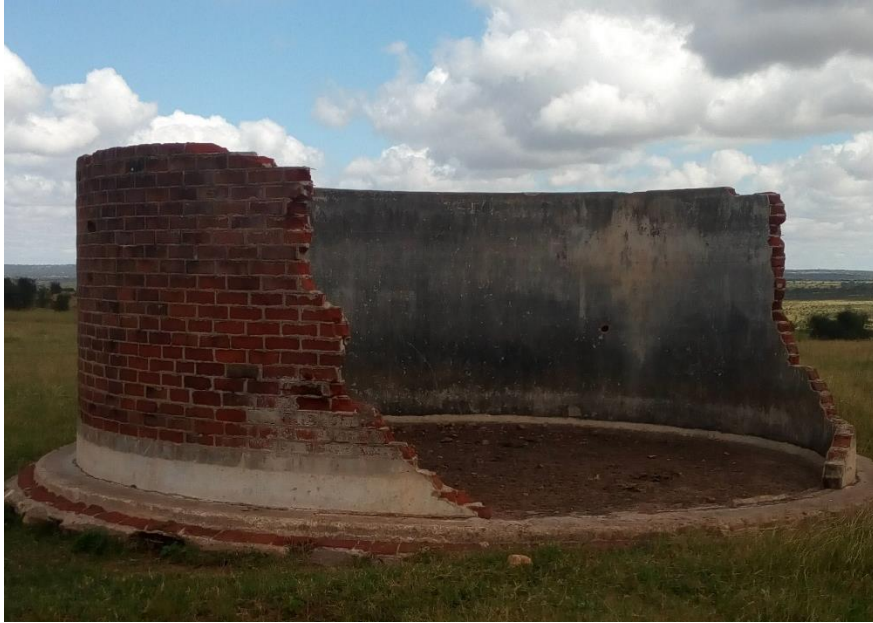
Figure 6: Destroyed Water Tank in AMK
