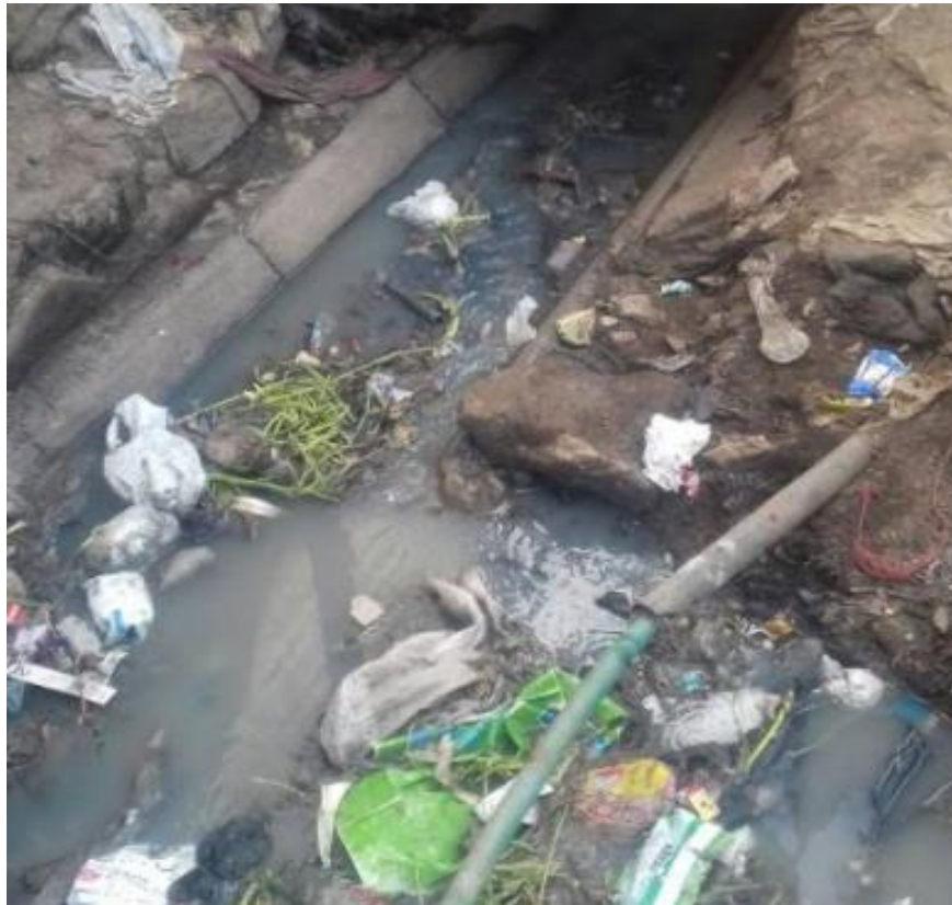
Figure 5.7: Storm water drain clogged by solid waste; water pipe nearby is at risk of contamination in the event of flooding
