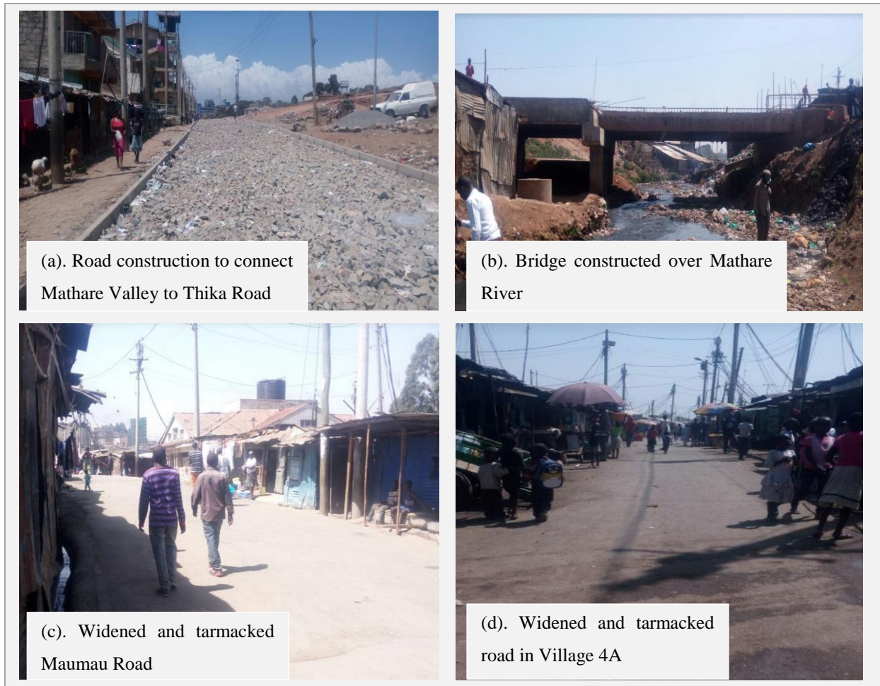
Figure 4.6: Various upgrading efforts across Mathare Valley: (a) road construction, (b) bridge construction, (c) and (d) road widening and tarmacking
