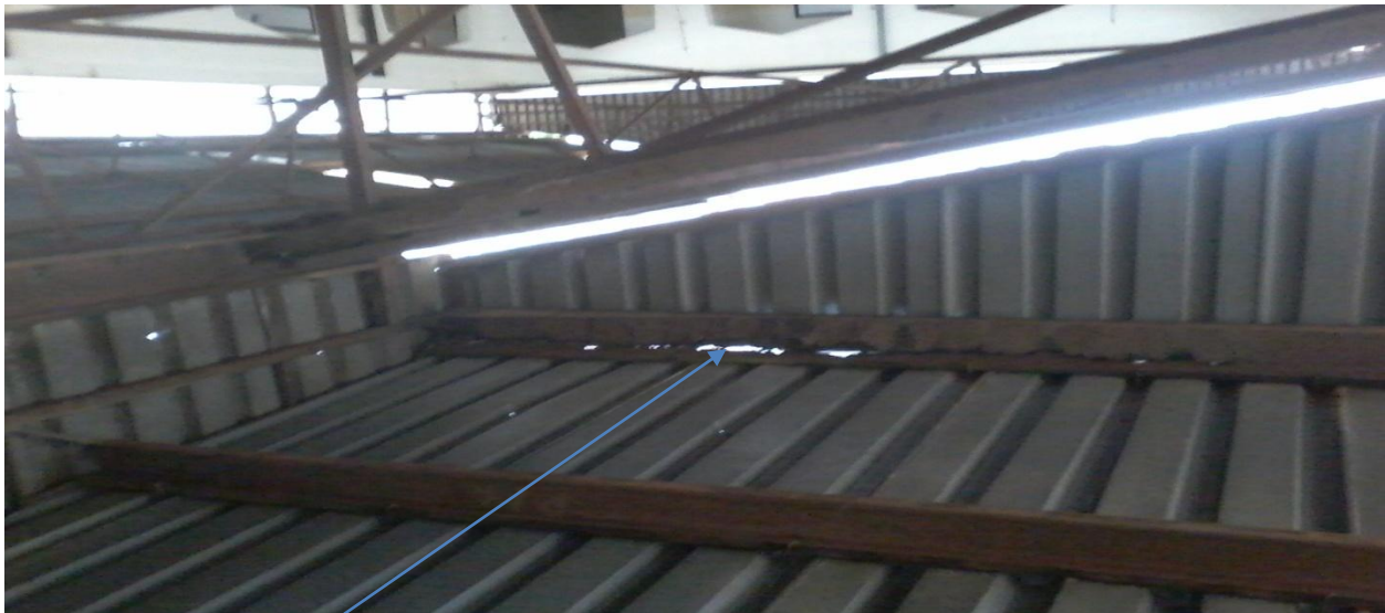
Figure 1.1: Corroded steel roofing rails
