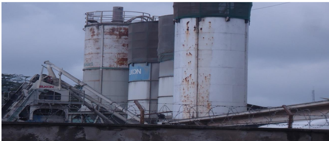
Figure 2.3: Metallic coated factory reservoirs with brown rust developed as patches
