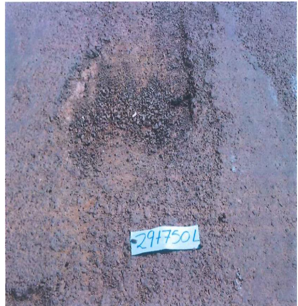
Plate 1.4: Ravelling of surfacing and pothole - Sigalagala-Butere Road (Source: Author, 2015)
