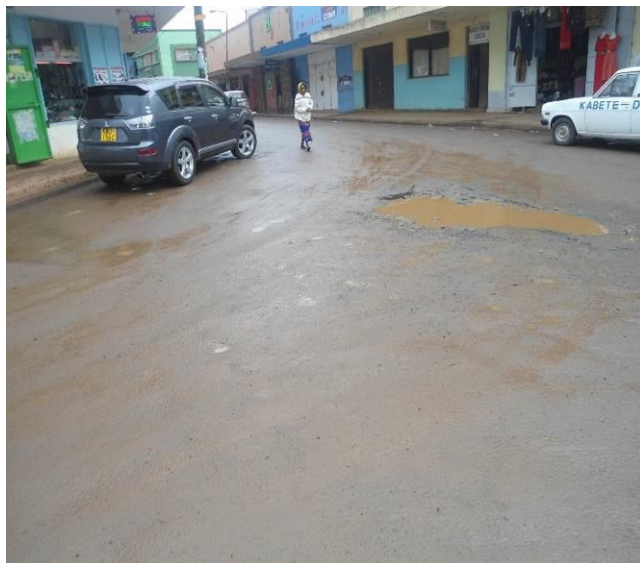
Plate 1.4: Potholed section of a Limuru township Road (Source: Author, 2016)
