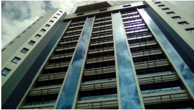
Figure 22: Glare Control in the UON towers using vertical and horizontal sun shading elements. Source: Author, 2018
