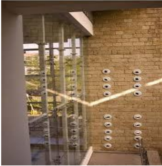
Figure 67: Cooling ducts in the Strathmore Business School building. Source: (Strathmore Business School, 2012)
