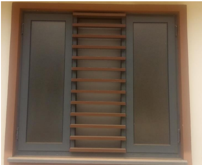
Figure 15: Windows showing wire mesh ventilation for permanent free air movement
