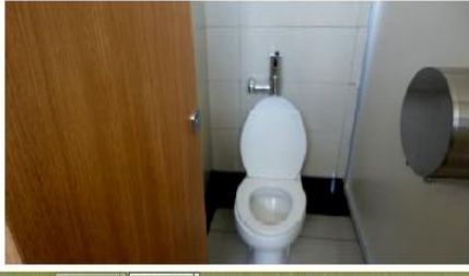
Figure 76: Water efficient toilets at the Strathmore Business School building.
