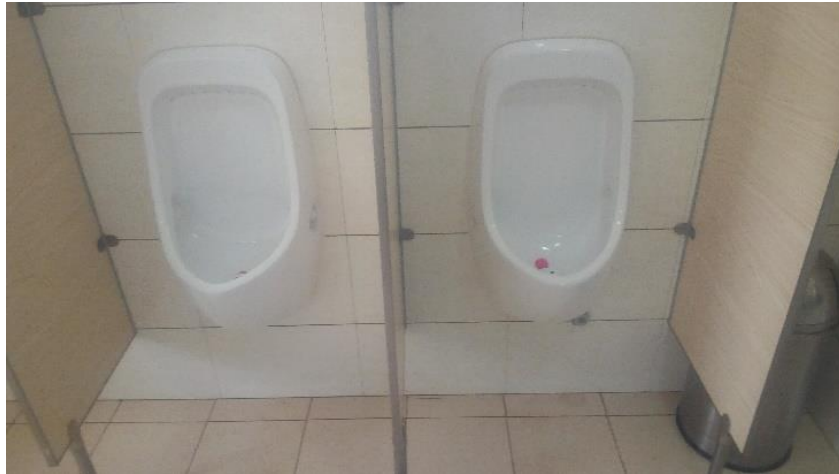
Figure 47: Environmentally friendly urinals in the building
