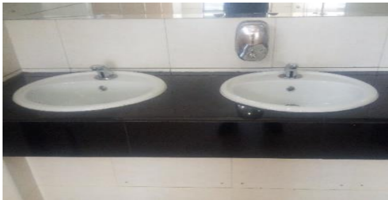
Figure 26: Some of water saving fixtures in the toilets Source: Author, 2018
