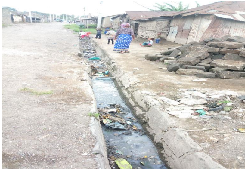
Plate 2: Poorly Maintained Drain
