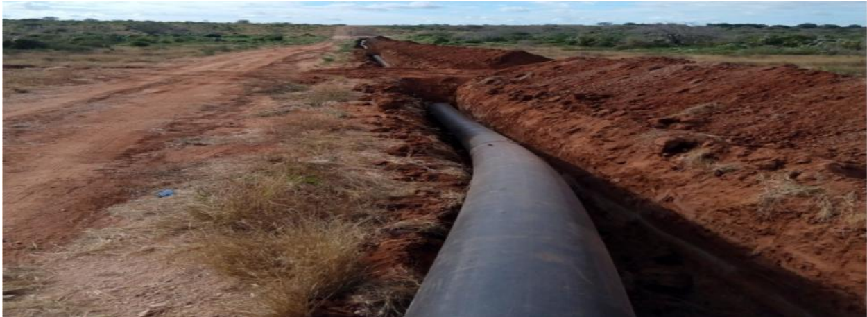
Figure 2: The main pipeline for the first drip irrigation area
