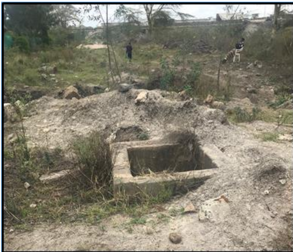
Plate 9: Open Manhole along Mtomawe Riparian
