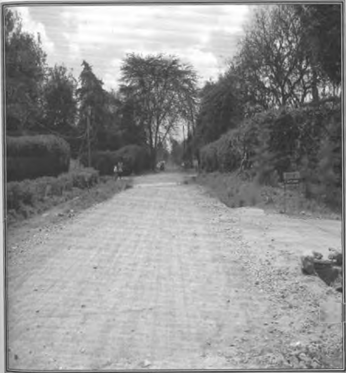
Plate 5.1: Poor state of Kiadaruma Road
