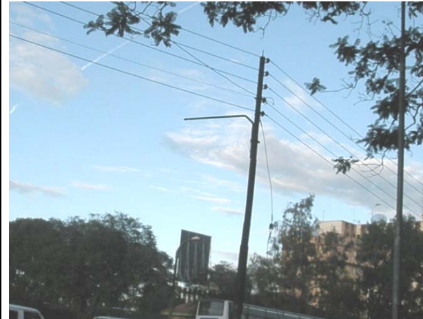
Some street lamps are in a state of disrepair
