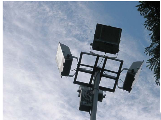
Tower security lamps, a close-up
